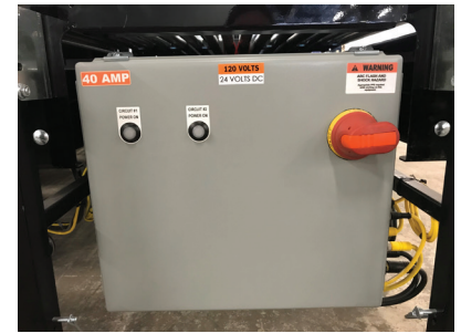
Figure 7: Power Panel with Disconnect Switch
